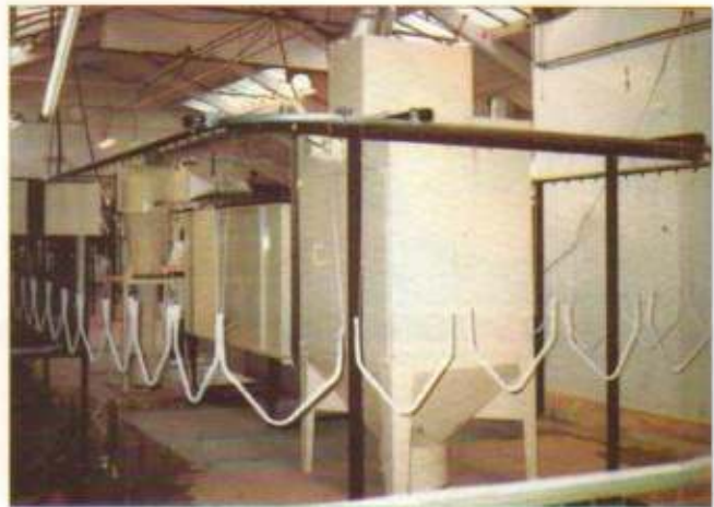
• Model 500 unpowered Turbaway cyclone and Dustaway model FWB375 as powder coating booth recovery system.
