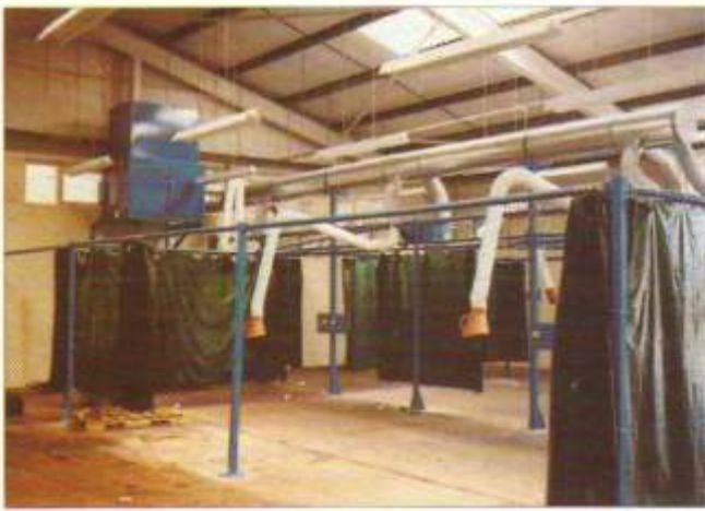
• Centralised welding fume extract system with wall mounted smokaway model FF6000 and extract arms Re-circulation of clean air.
