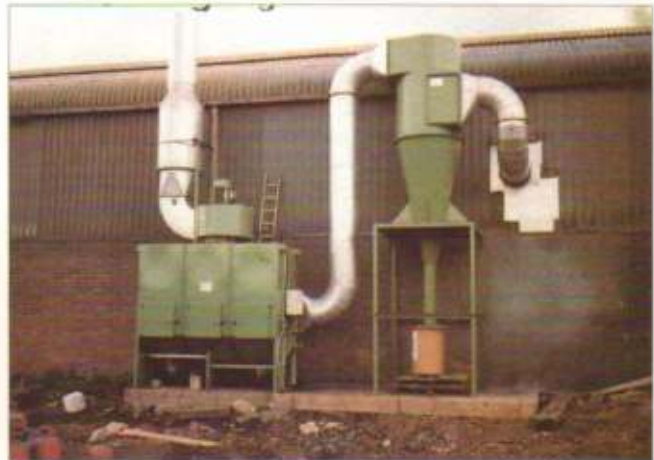
• Model 900 unpowered Turbaway cyclone in Zinc spraying operation.
