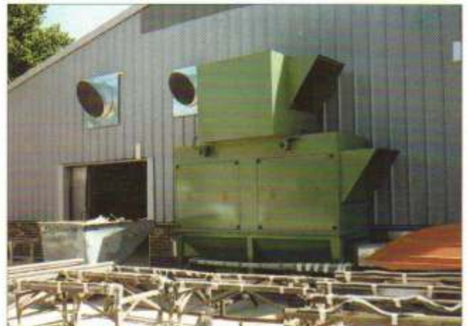
● Dustaway model FWB1200 units shake on trim room building.
