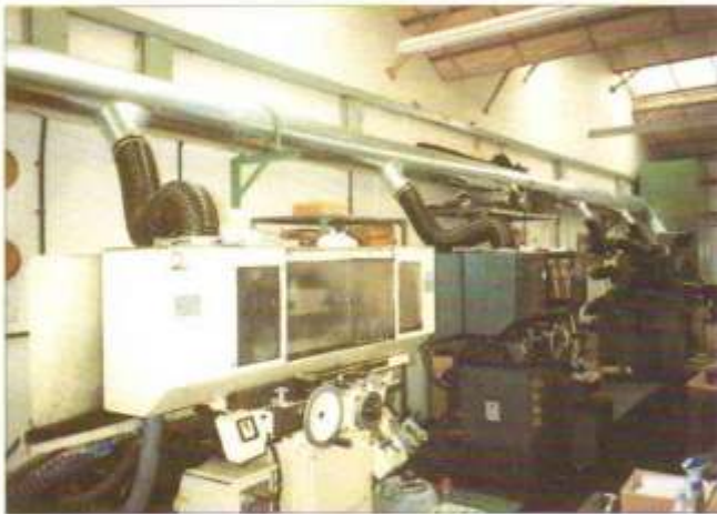
• Centralised extract system for wet machining operation with Mistaway model MF6800 filter unit. Re-circulation of clean air.
