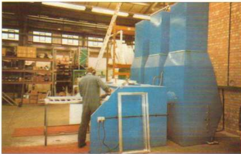
● 9'0" wide low profile fettling booth and three model W2000 self induced wet dust collectors.
