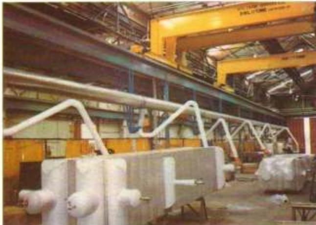
• Large centralised welding fume extract system to atmosphere using 4 metre long extract arms.
